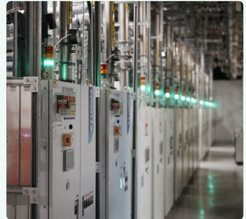
TSMC enhances standby mode for electric-heating local scrubber backup units.
