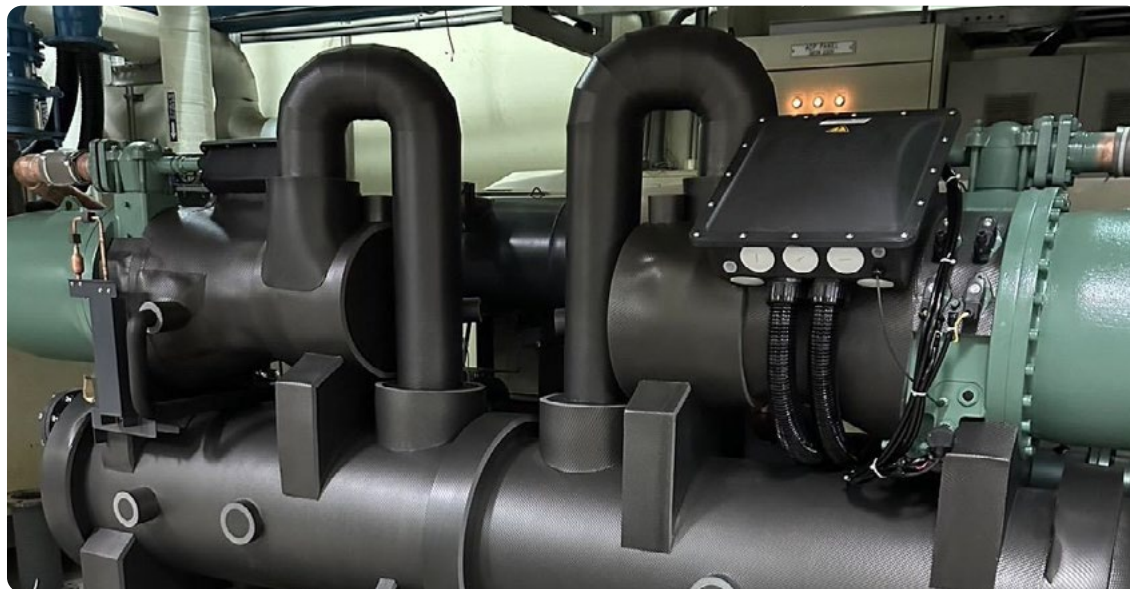
TSMC subsidizes suppliers in upgrading chiller systems
