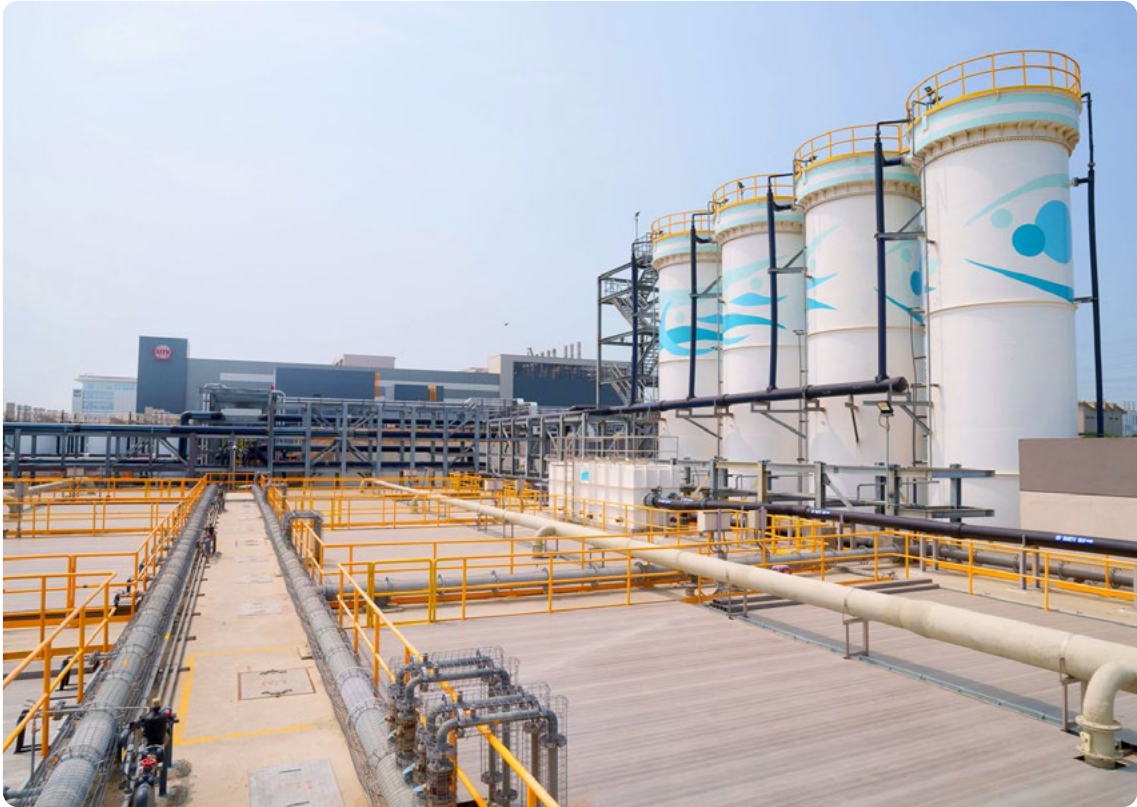
TSMC S.T.S.P. Reclaimed Water Plant
