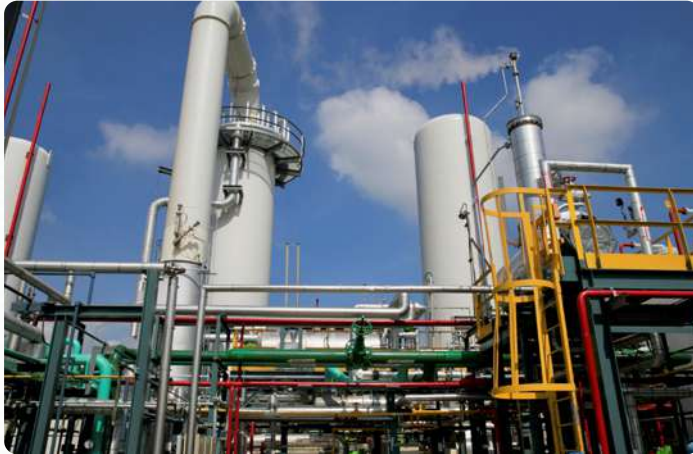
The supplier installs a carbon dioxide recovery and purification system in the hydrogen production plant.
