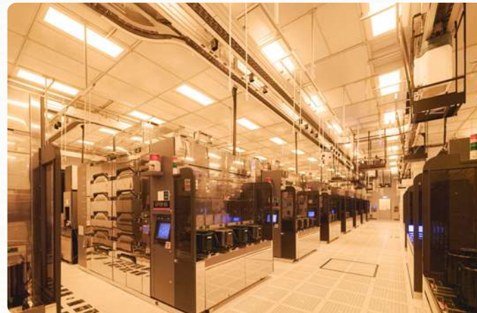
TSMC collaborates with suppliers to improve operational efficiency of power transformers.
