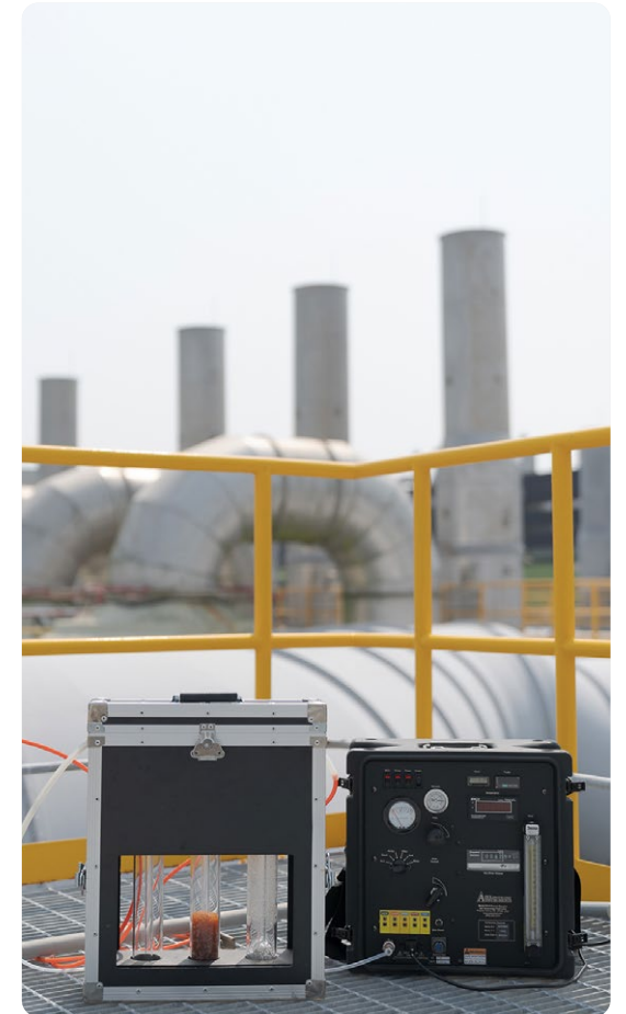
TSMC reinforces the monitoring capabilities of its air pollution control equipment.
