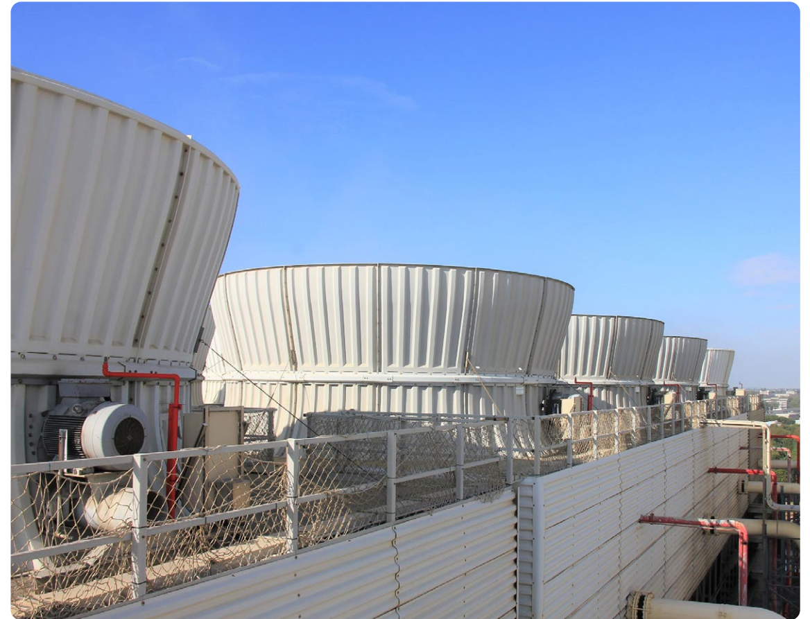
▲ TSMC continues to develop energy-saving and carbon-reduction measures, enhancing energy efficiency.
