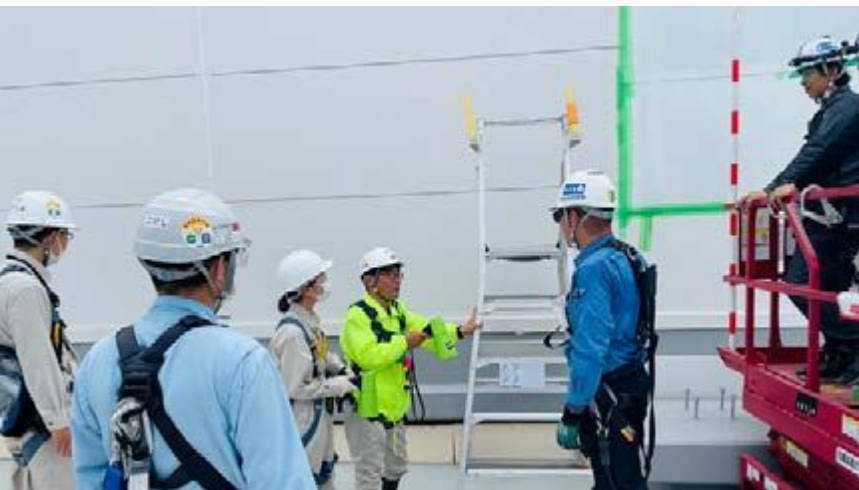
TSMC collaborates with third-party safety experts to implement the Construction Safety Management Counseling Project
