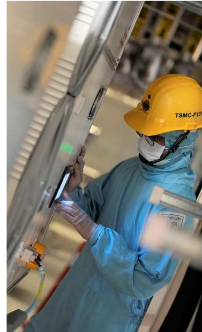
TSMC retrofits the hot DI water circulation system of wafer cleaning tools to expand energy saving benefits
