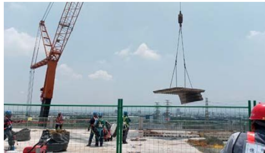
Full-time monitoring of high-risk operations by dedicated personnel
