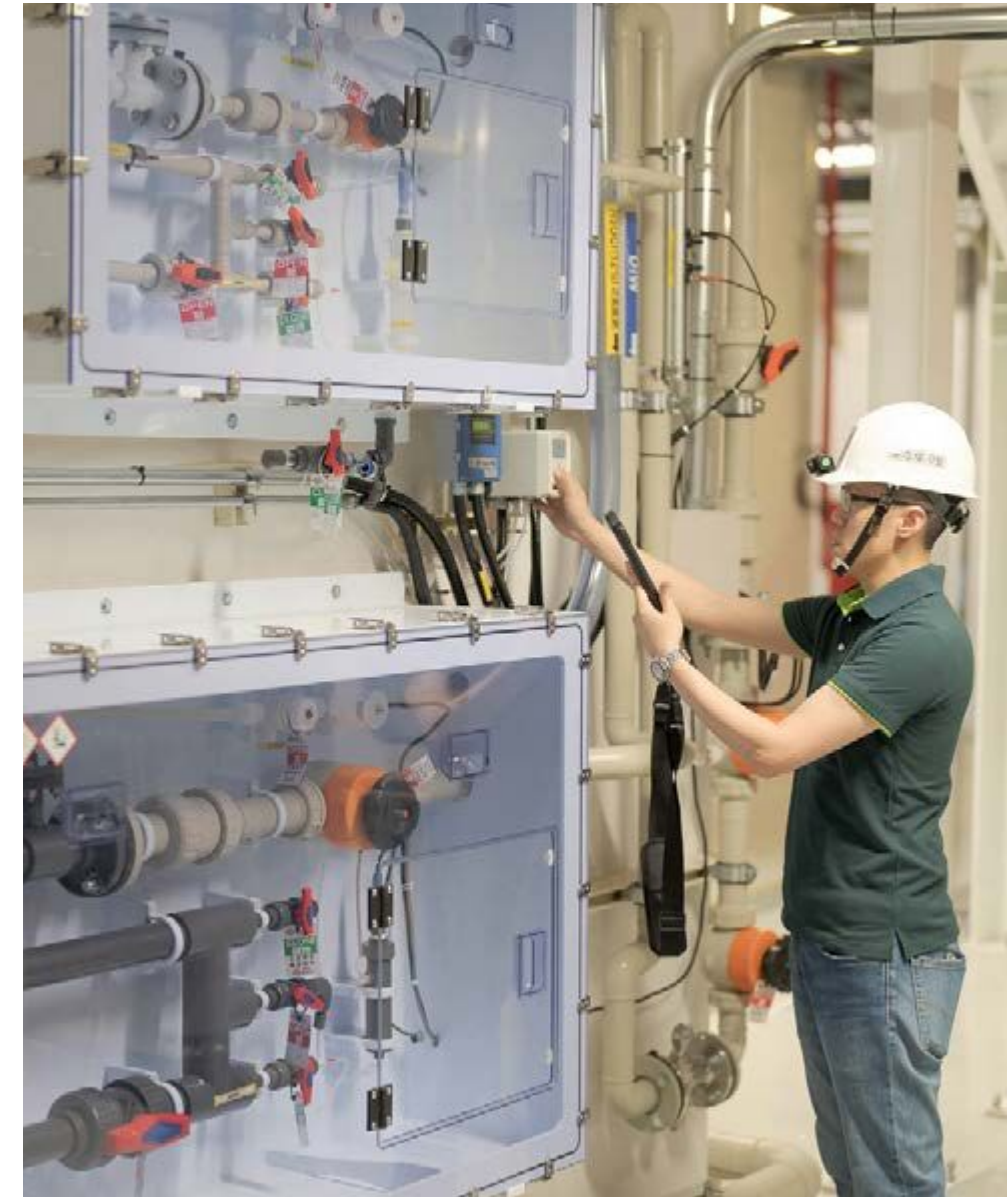
TSMC innovates HOCl Conversion System to reduce chemical consumption
