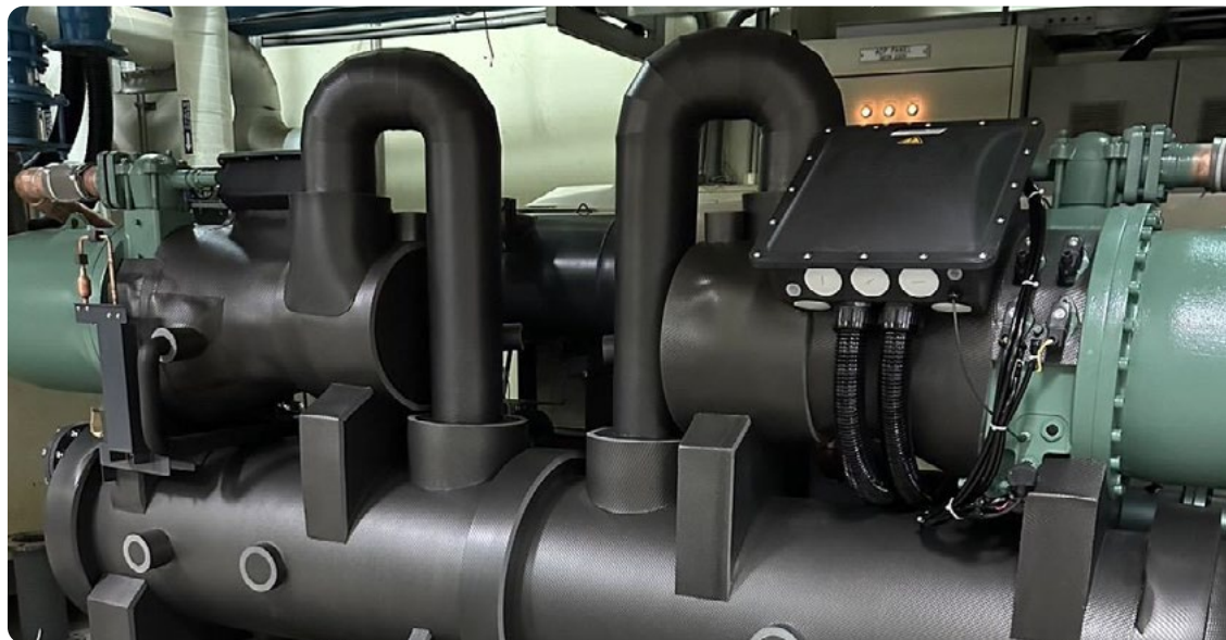
TSMC subsidizes suppliers in upgrading chiller systems
