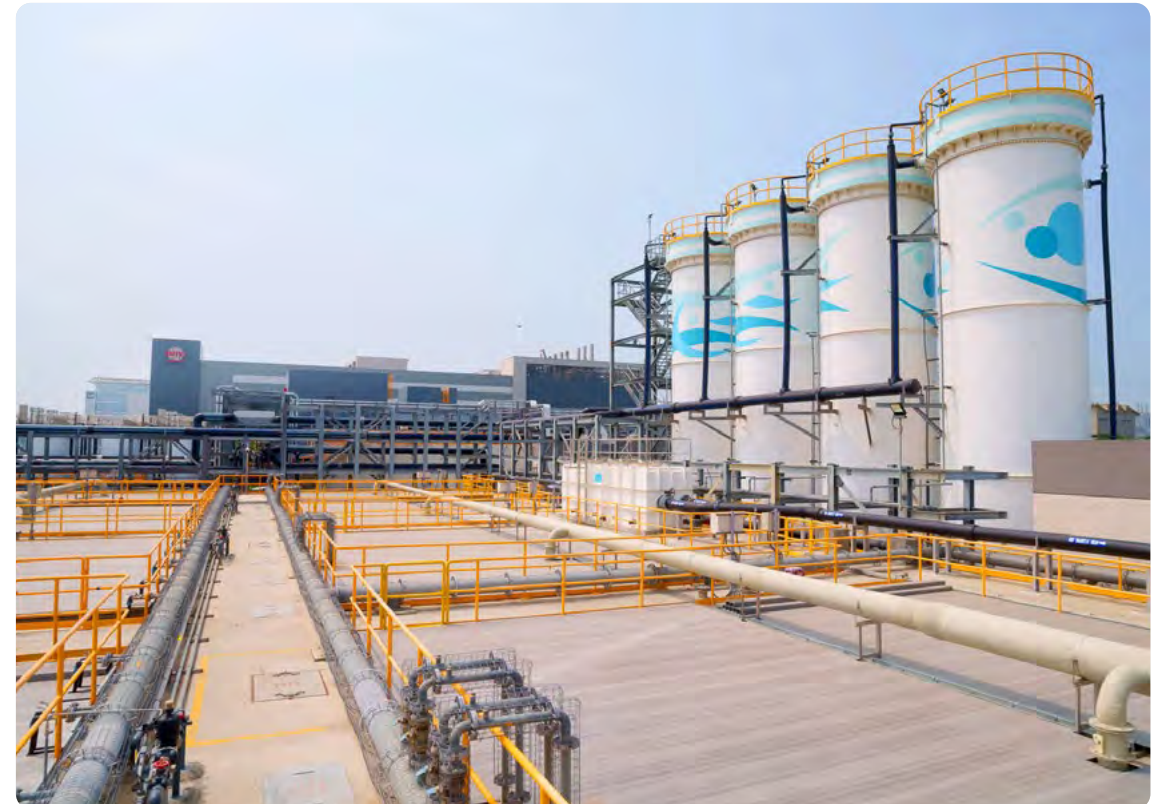
TSMC S.T.S.P. Reclaimed Water Plant
