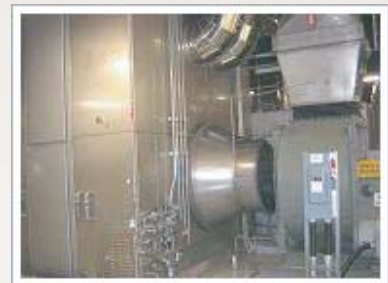
VOCs pollution control facility - Zeolite Concentration Rotor
