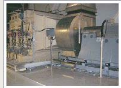
Acidic gases pollution control facility -Wet Scrubber
