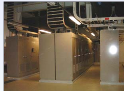
Inverters in Process Water System
