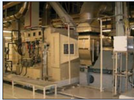
Acid gases pollution control facility – Wet Scrubber
