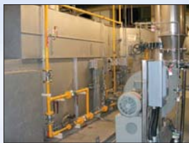
VOCs pollution control facility – Zeolite Concentration Rotor
