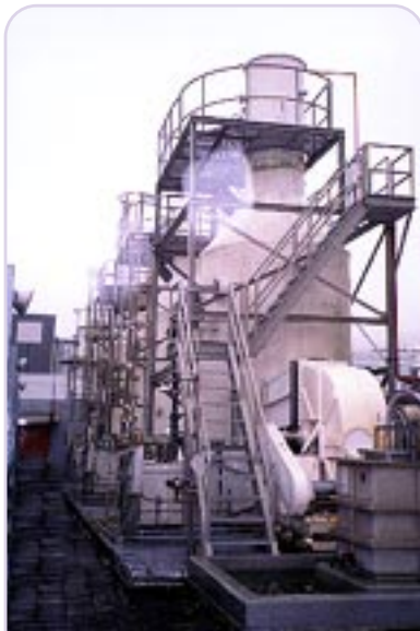
Acid & Alkali gases pollution control facility - Wet Scrubber
