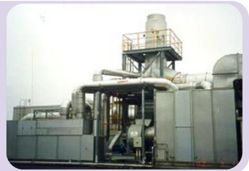
Volatile Organic Compounds (VOC) pollution control facility - zeolite concentration rotor
