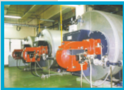
High efficiency natural gas boiler
