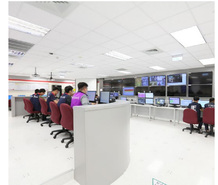
Facility Monitor Control Center
