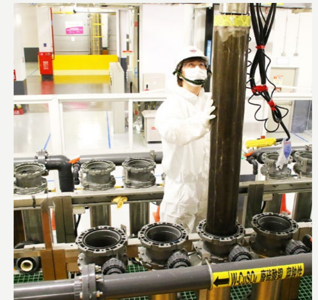
Copper Wastewater Recycling System
