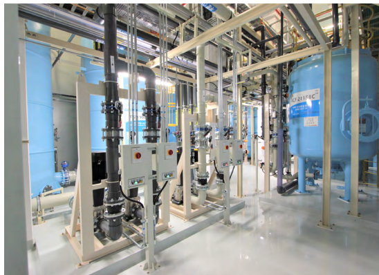
Fab 18A biological treatment system.
